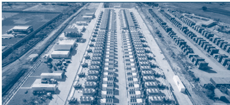
Figure 3. Close Up Of The Installation In Myanmar
